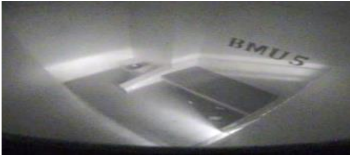
Photograph 1: BMU cell 5, taken from CCTV footage
